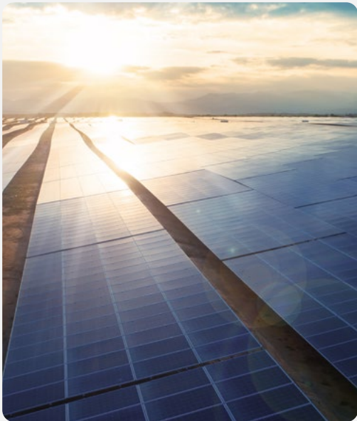
Solar panels on the 405 MW Ninh Thuan solar farm in Vietnam owned by ACEN
